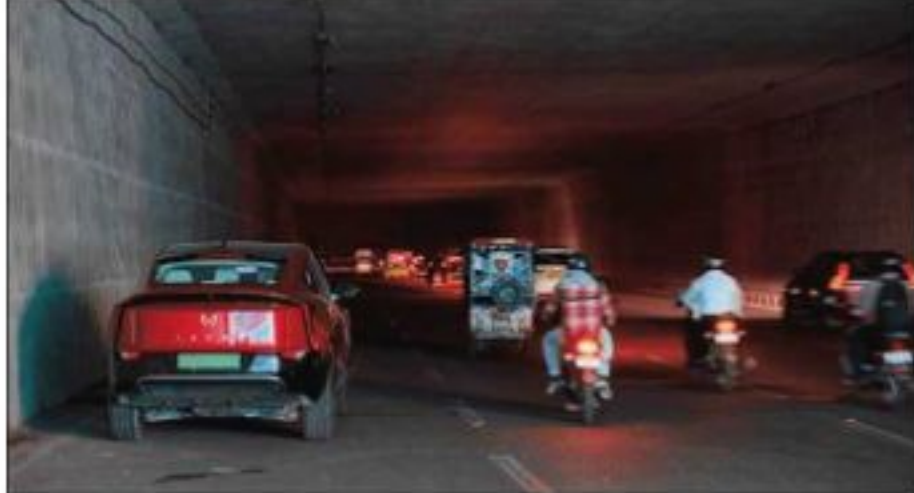
Commuters using the underpass on the Delhi-Gurgaon border have been navigating the stretch in darkness for the past two days
